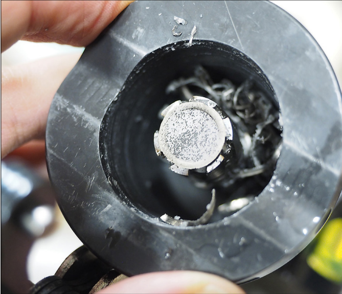
After drilling EACH hole, inspect the cutter assembly. Check for a slug and shaving build up (present in the above image).
