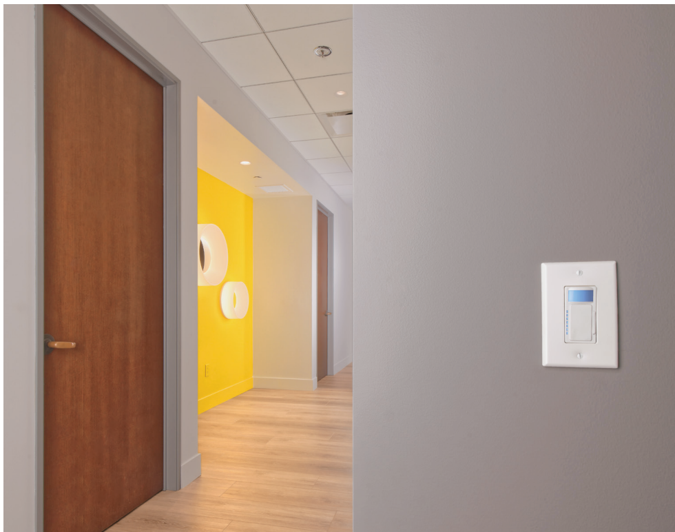
Figure 5. The project team was able to remotely commission the control network to maintain progress during the statewide Covid shutdown.
